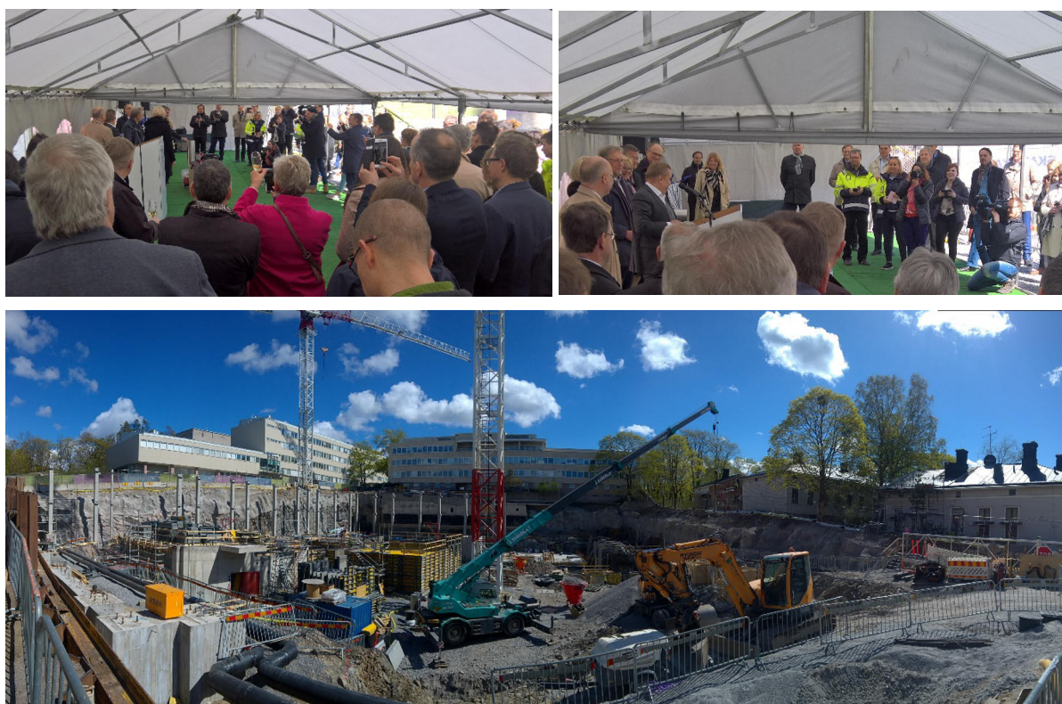
Laying the foundation (Grundstensmurningen) 8th of May 2019. Speeches by the mayor of Turku, Minna Arve and the university rectors Mikko Huuza and Kalervo Väänänen.
