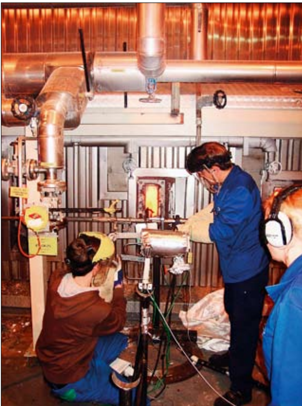
Measuring gas composition inside a boiler
