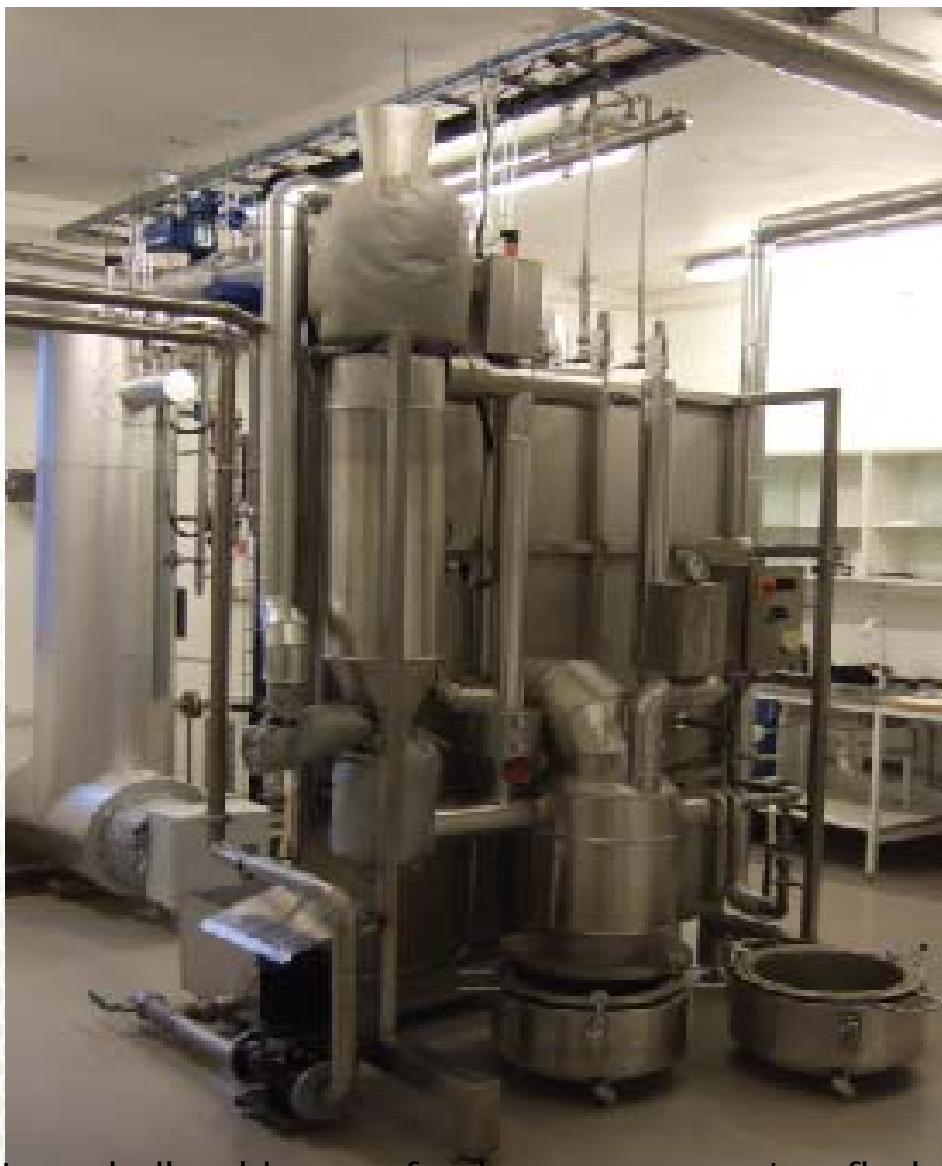
Steam boiler, biomass feed, pressure reactor, flash tank,
